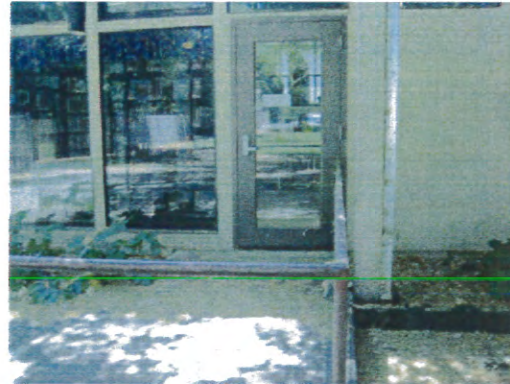
Emergency egress door. Compliant hardware and side access
