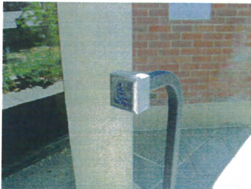
Auto door opener location, height and access compliant
