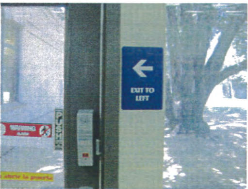
Exit Route signage is not clear or consistent. Recommend revising any signs referring to path of exit and add Braille signage for Exit Route
