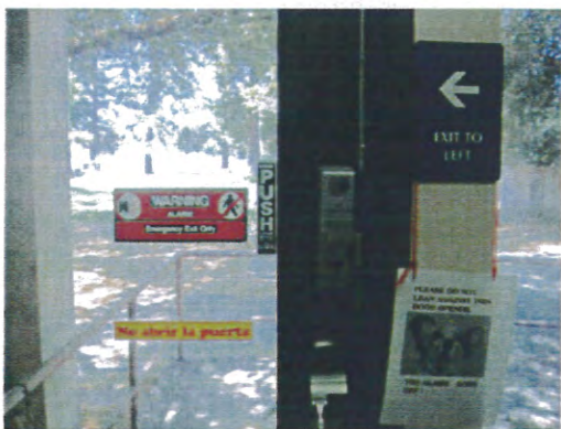
Exit Route signage is not clear or consistent. Recommend revising any signs referring to path of exit and add Braille signage for Exit Route
