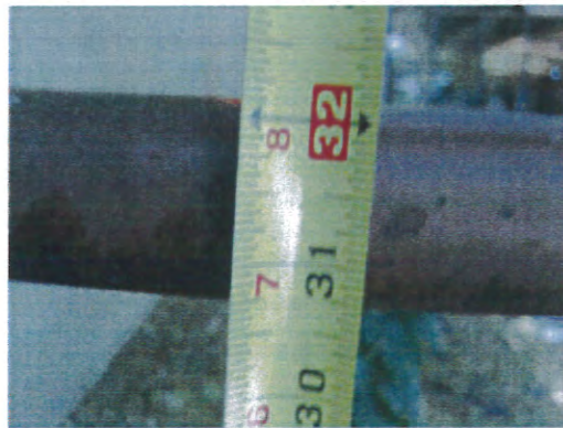
Ramp rails no compliant with height, wheel guides or rail extensions
