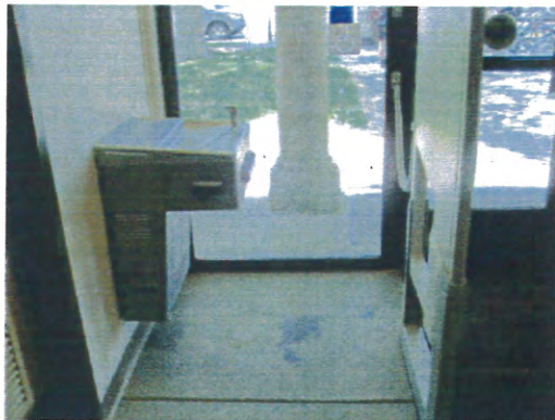
Drinking fountain not accessible to the disabled. Alternate water cooler provided
