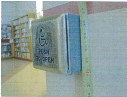
Location in auto door opener compliant for access and reach
