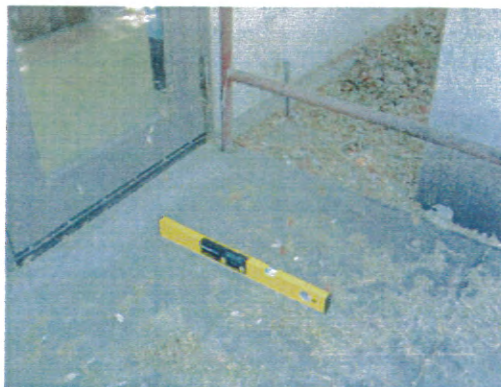
Landing running slope not compliant at more than 2%
